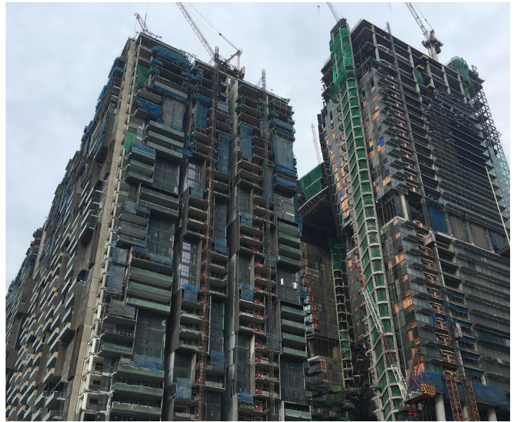
Singapore construction tipped to speed up this year. Source: S&P Global Platts
